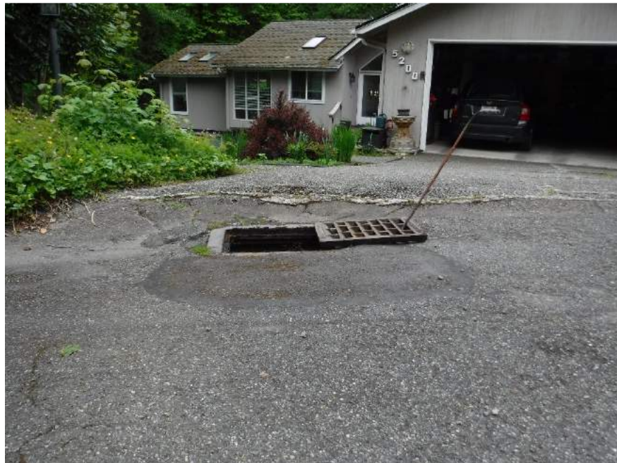
Image 4: Downstream flows are conveyed to this CB via a 12" concrete pipe
