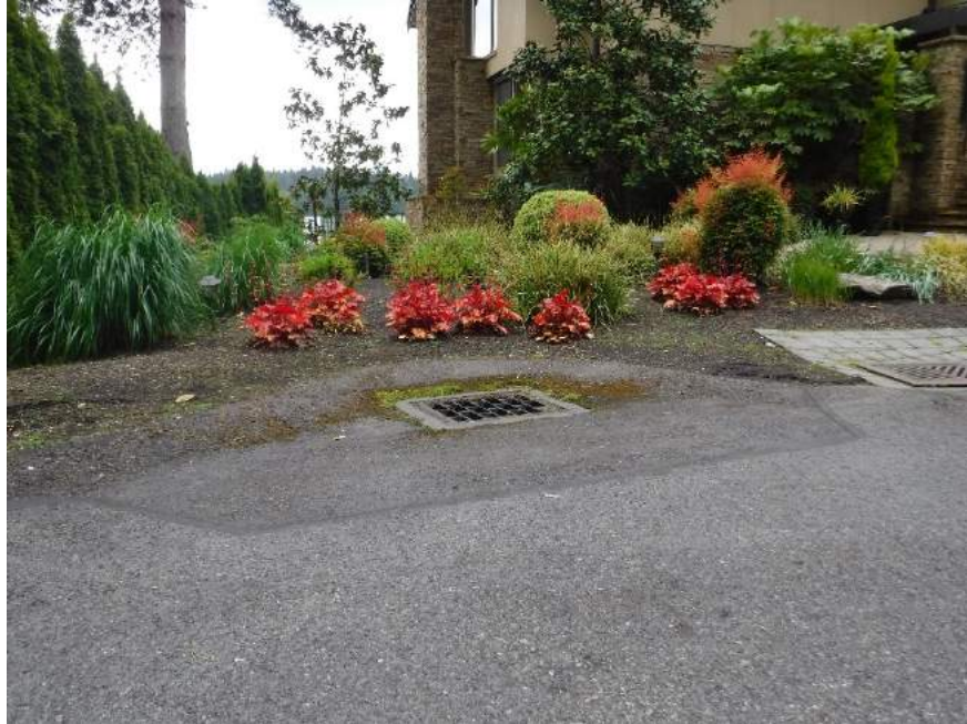
Image 9: 24" concrete culvert pipe enters this CB and flows continue in the westerly direction via 30" corrugated aluminum pipe through a private drainage easement located at 5067 SE 51 st St
